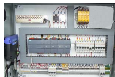
Typical Touch Screen Operator Interface. Siemens S7-1200 PLC with Ethernet Interface and DSL Router.
