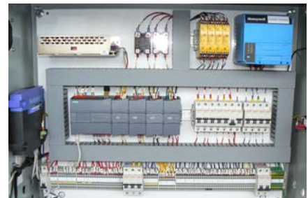
Standard Control Panel with Siemens S7-1200 PLC, Safety Relays, automatic circuit breakers, Ethernet Router, and Honeywell Flame Safeguard.
